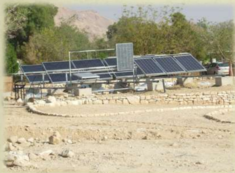
Capital Nature AIES Solar Energy Technology Validation Center
